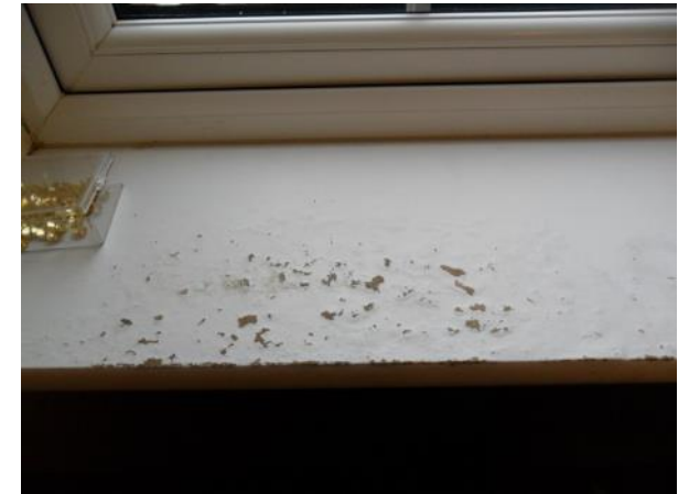
Chipped paint to window cill
