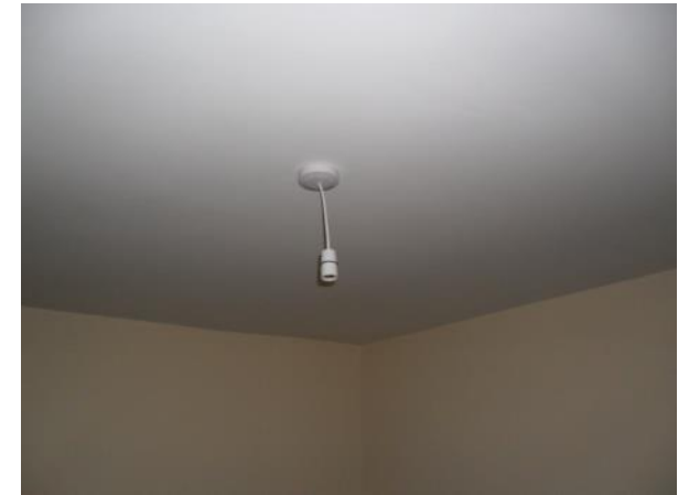
Missing bulb to light fitting
