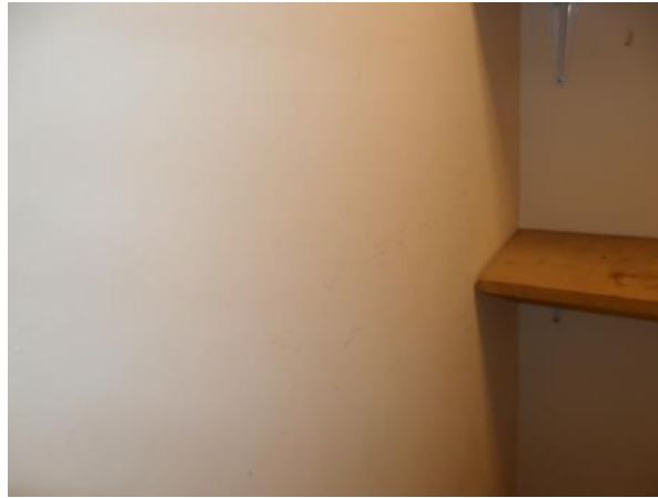
Minor scuffs to Wall
