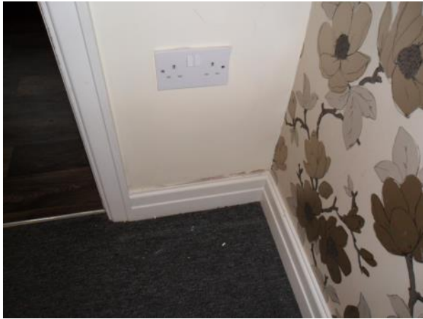
Chipped paint to Wall
