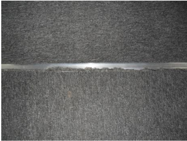
Carpet loose/come away from threshold
