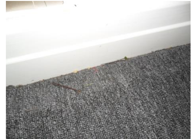
Dirt to edge of carpet
