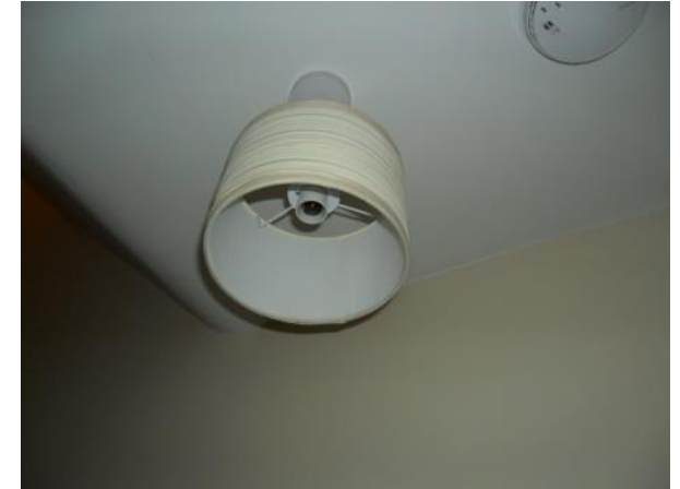
Light fitting with missing bulb
