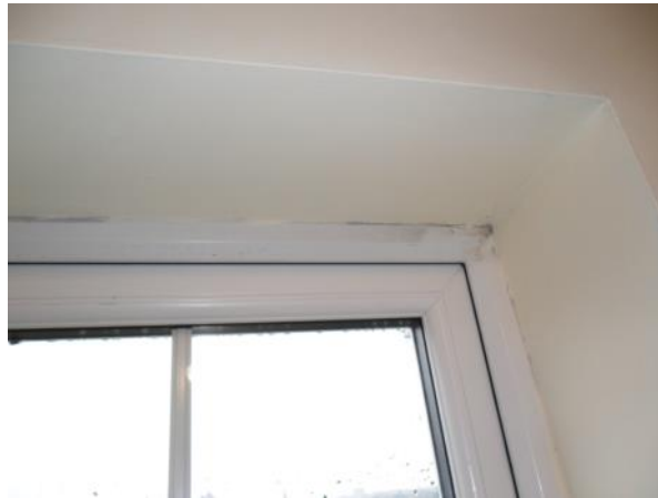
Dirt to Kitchen window
