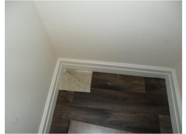
Missing Vinyl to conrer
