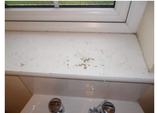
Chipped paint to window sill in bathroom
